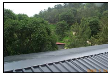
Close-up of rooftop panels and the surrounding Costa Rican countryside.
